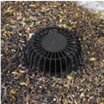
Clogged drainage openings
