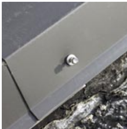
Loose flashing screws
