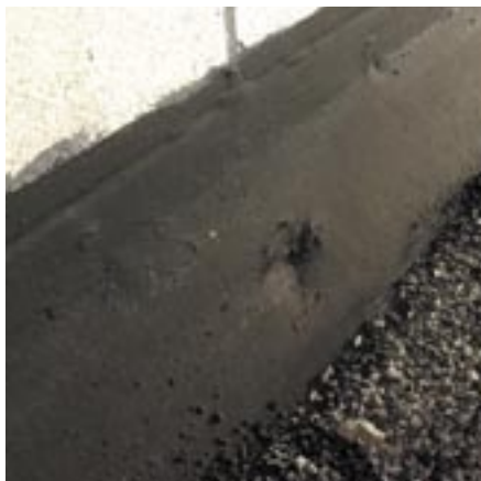
Punctured wall flashing
