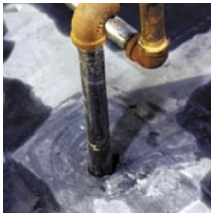
No roof flashing at new gas pipe penetration
