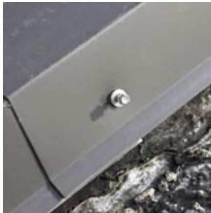
Loose flashing screws
